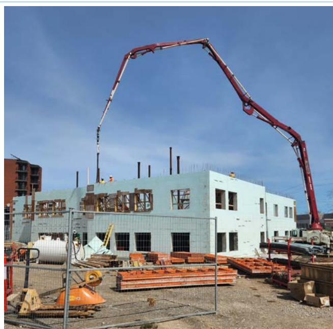
Construction of the second storey of the Long-Term Care Home’s new East Wing.
